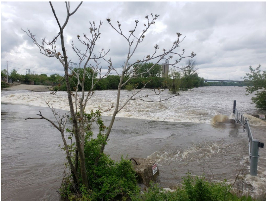
Photo 2: Picture of water flowing over the low water crossing road on the way to the Cargill boat ramp. The picture was taken May 18th, 2020, looking south-southeast.
